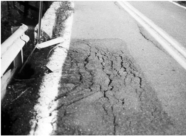
Cracks and settling in asphalt indicate a failing culvert.
