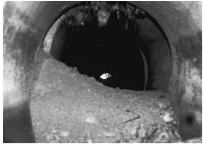
Silt filling this culvert drastically cuts flow capacity.
