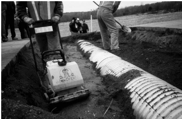
Adequate compaction is essential to culvert installation. Hand tamping is often best.
