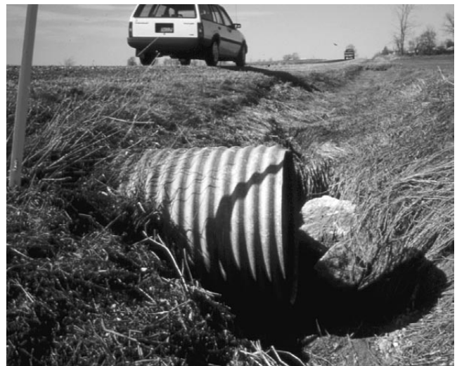
Erosion, a sign of inadequate capacity, has undercut the end of this culvert pipe.
