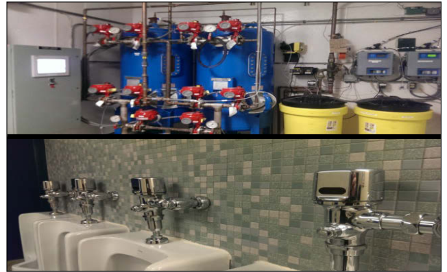
Treatment equipment & fixtures at Sterling Elementary
