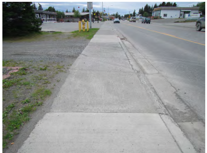
Figure 20: Driveway Entrance with Steep Cross Slope
