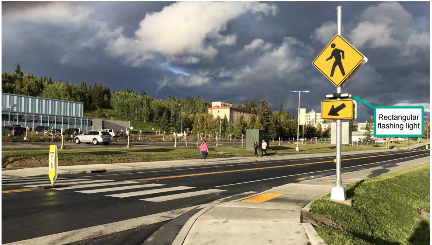
Figure 21: Electrical Warning Devices (Rectangular Rapid Flashing Beacon, or RRFB) on University of Alaska Fairbanks Campus
