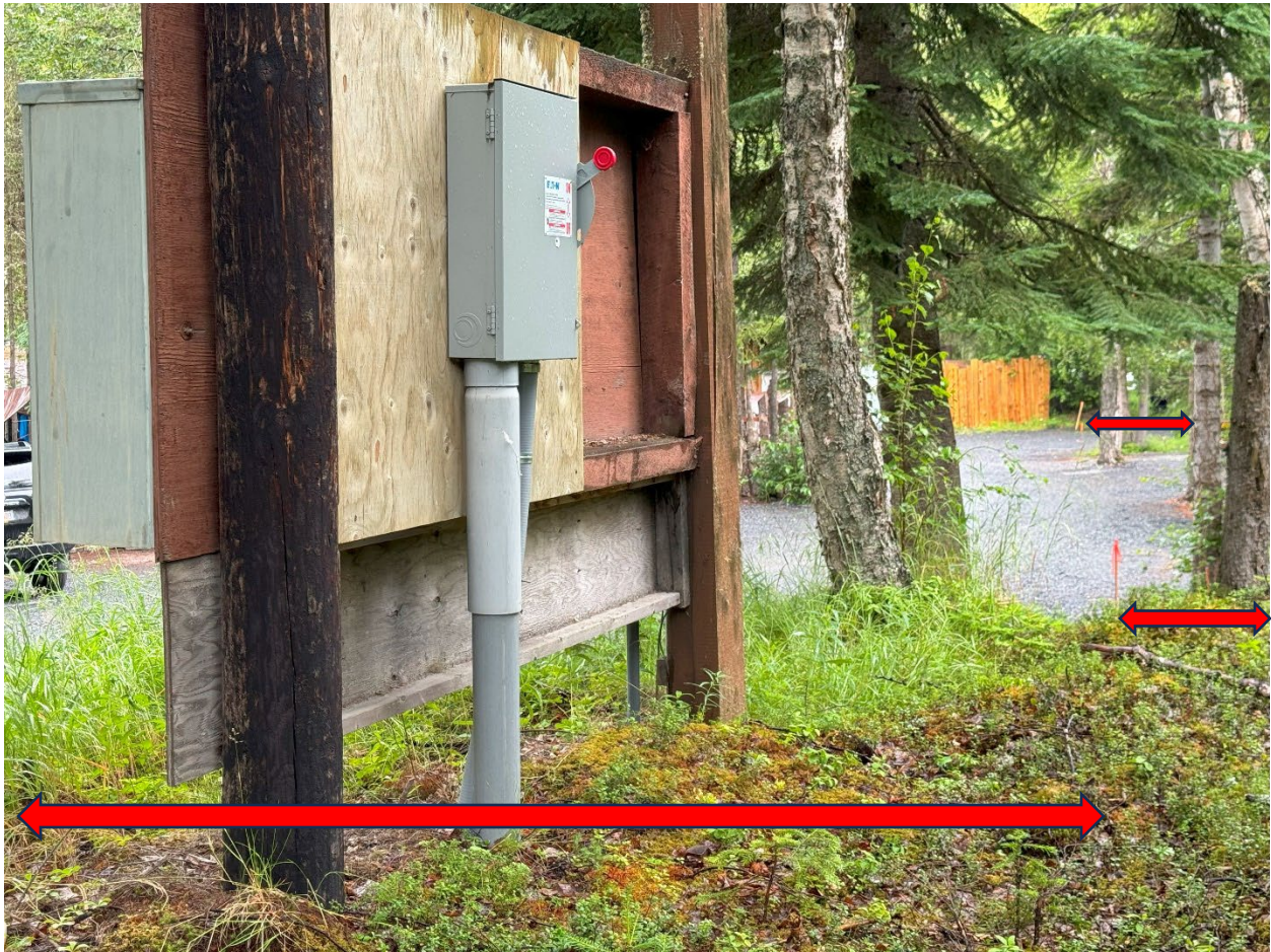
Annotated arrows from visible property edge stakes are approximate and illustrative only. Main utility pole and meter base has been in continuous operation since before the ROW was platted.
