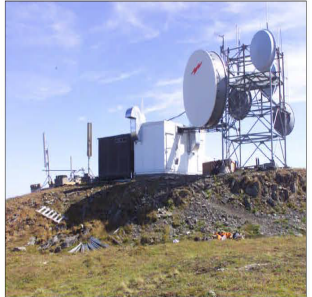
1 Cooper Mountain Communication Site
