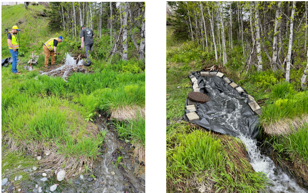
Figure 2. Site of collapsed pipe and associated manhole.
