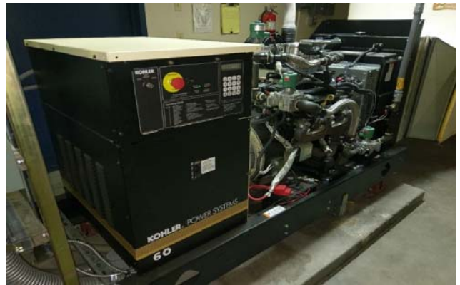
Emergency generator at Kenai Central Auditorium
