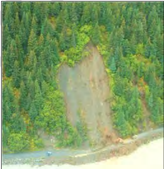
Lowell Point Road Landslide (2012)
