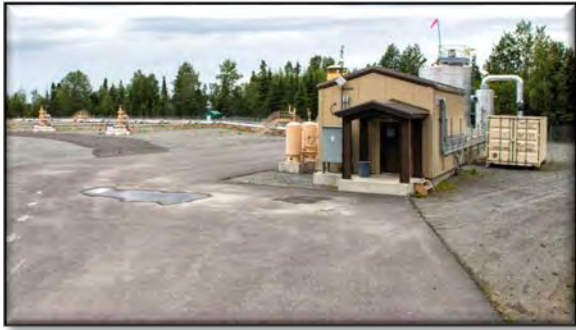
Gas Facility in Kenai
