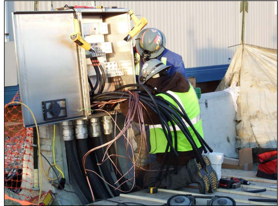
Electrical panel for microturbines
