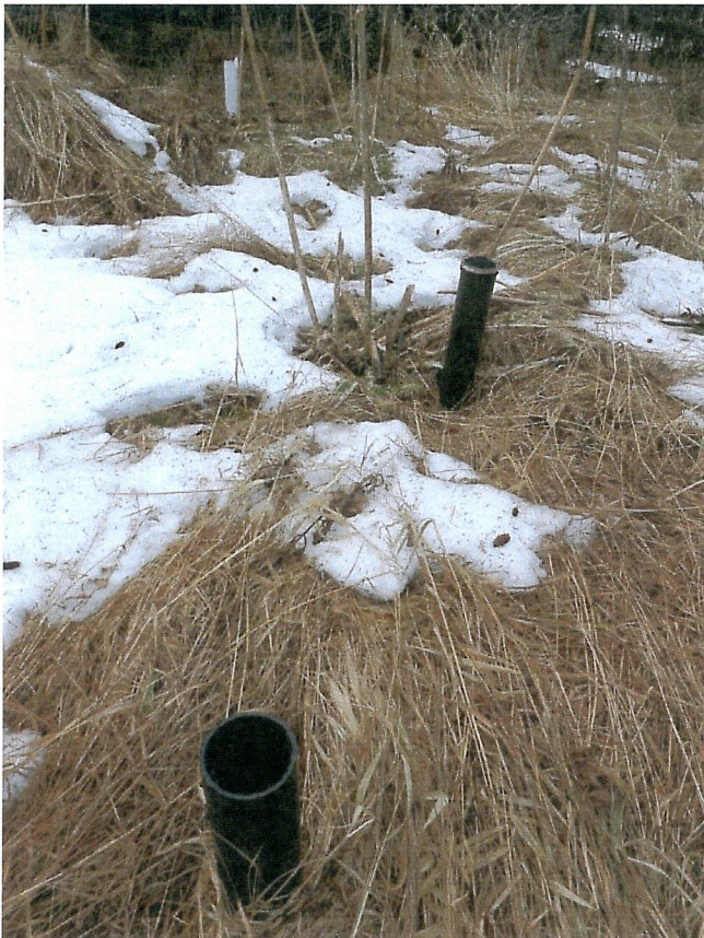
Photo 2: Septic Tank Risers (with missing caps)
