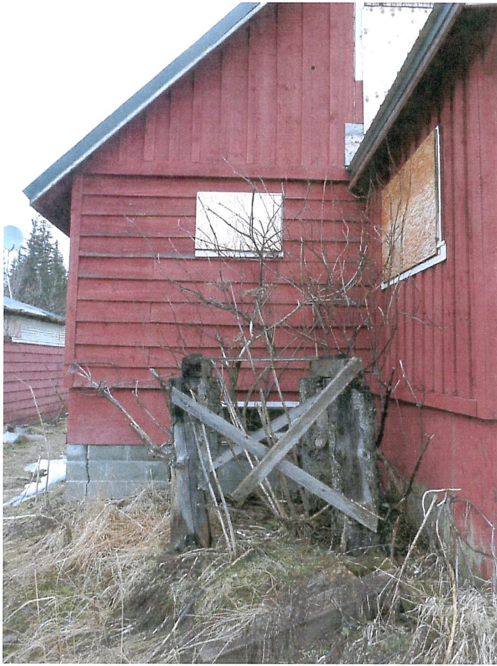
Photo 7: Fuel Tank Stand on Backside of House
