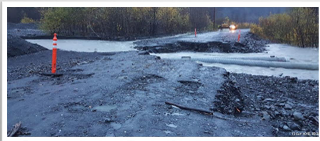
Japanese Creek overwhelms Dieckgraeff Road culverts during 2018 flood event.
