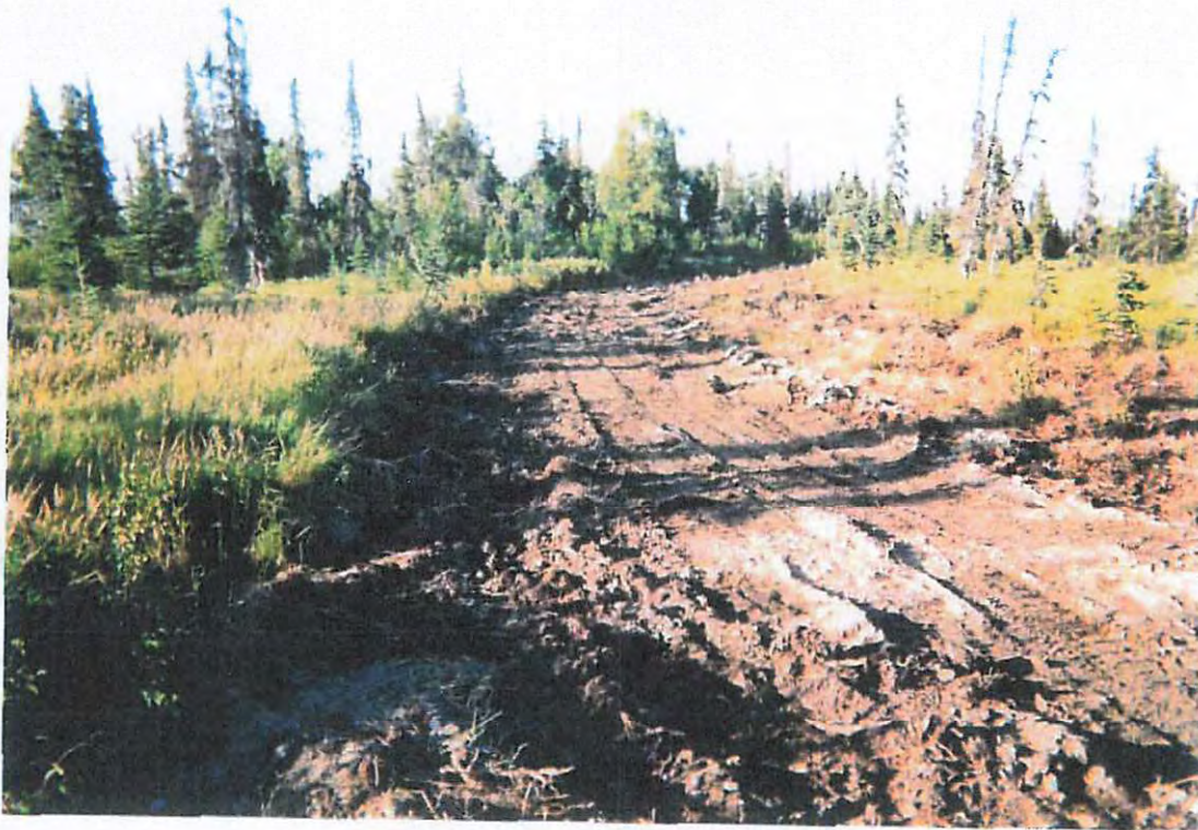
United States v. Abelgaard, et al Photo No. 3 August 2005 Rowan Circle restoration; view north, west shoulder
