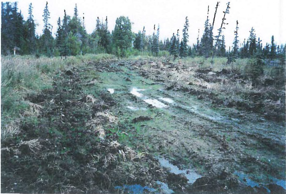
United States v. Abeldgaard, et al Photo No. 27 Aug. 29, 2005 SWPPP Inspection--Rowan Circle revegetatation; view north
