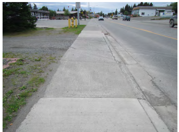
Figure 20: Driveway Entrance with Steep Cross Slope
