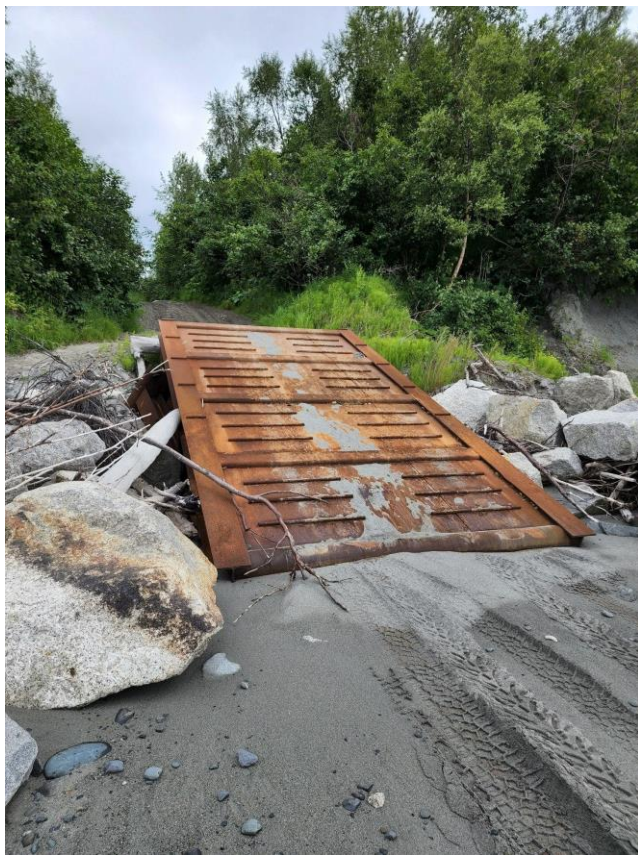
Current beach access at Pig Station, ramp is estimated 45° angle
