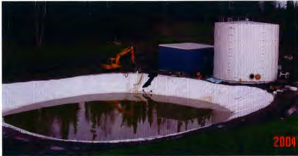
CPL Leachate Storage Tank and Lagoon
