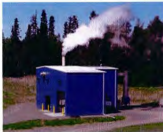
Leachate Evaporator System & Building (2014)
