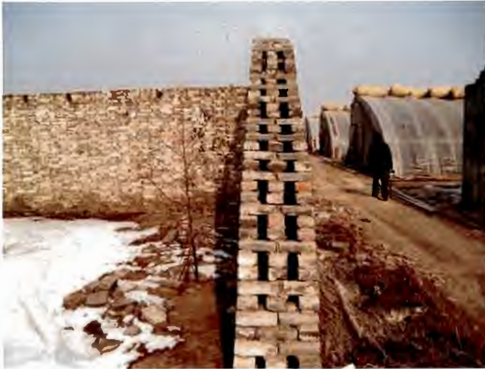
Air cavities in a ruined solar greenhouse. Picture: Chris Buhler, Indoor Garden HQ.
