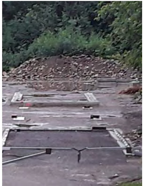
Figure 2: Standing Water at STT Site
