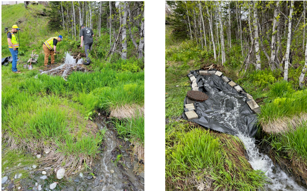
Figure 2. Site of collapsed pipe and associated manhole.
