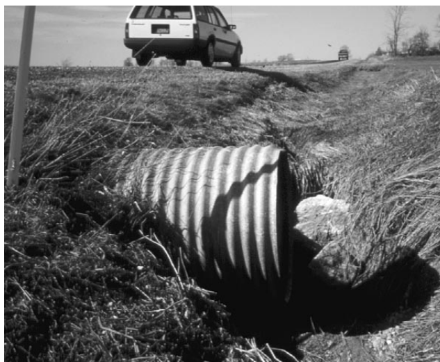
Erosion, a sign of inadequate capacity, has undercut the end of this culvert pipe.
