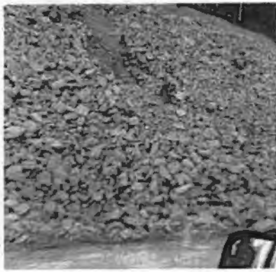
Above, sloughing rip rap below Ravens View, Geoff Coble and Ken Green, March 12 looking down to Snug Harbor Road. Right, included in Coble's report is picture of 1986 slope failure near Senior Haven. The liquefied earth went through a power line and took down trees on the way to Snug Harbor Road. CLSCCI knows the importance of drainage under and near the apartment buidlings!
