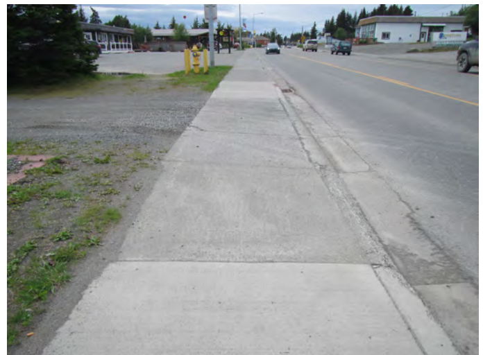
Figure 20: Driveway Entrance with Steep Cross Slope
