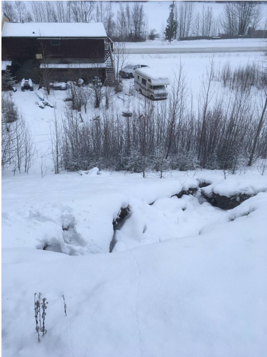
Photograph #4: Failed slope from above.
