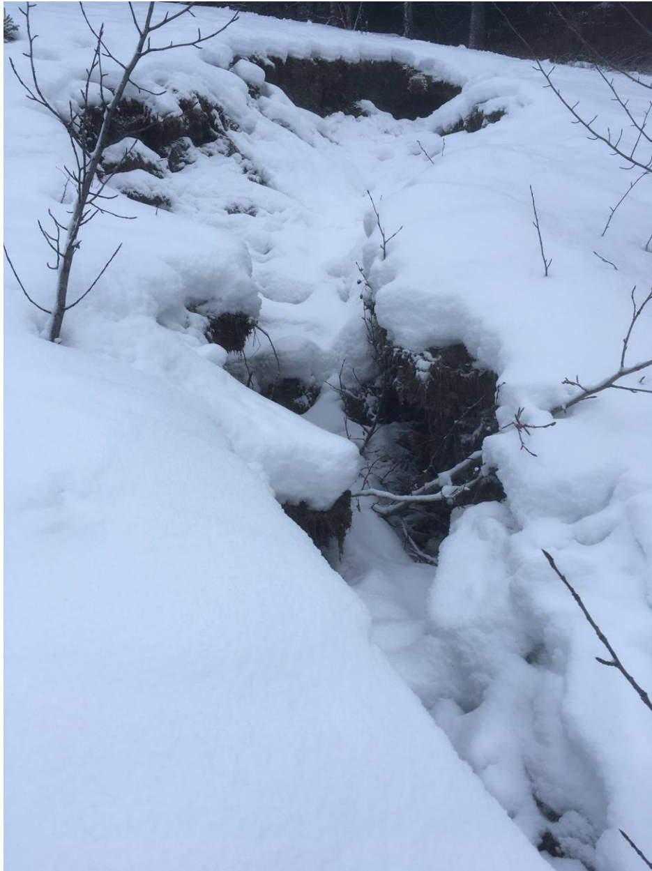
Photograph #3: Failed slope from below.
