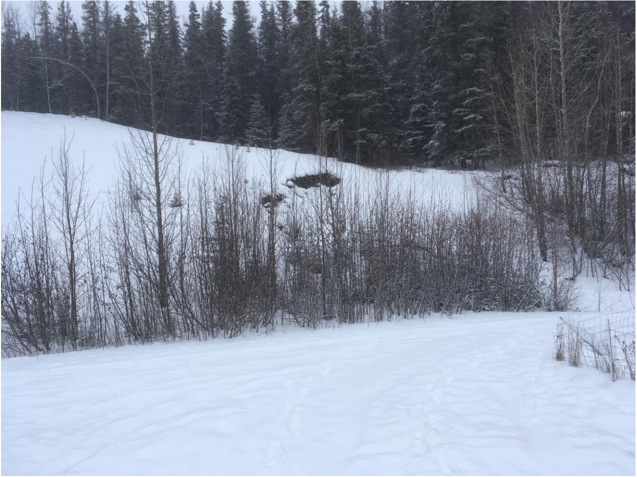
Photograph #2: Area of failed slope.
