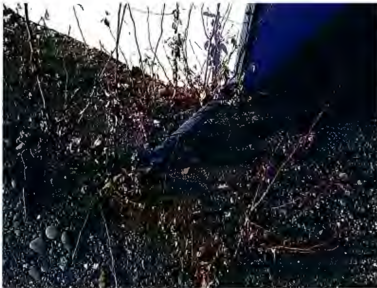
Phot 3: Crushed downspout extension.
