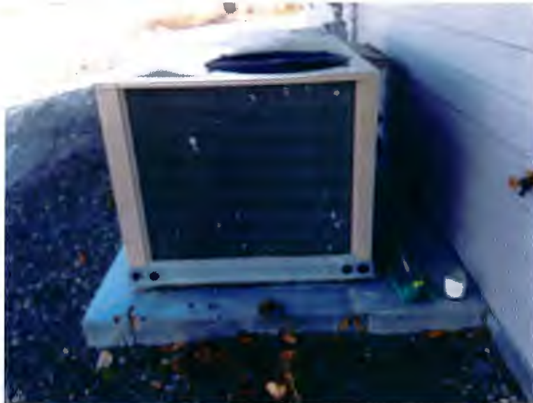
Photo 5: Gas fired, ground mounted, package HVAC unit.
