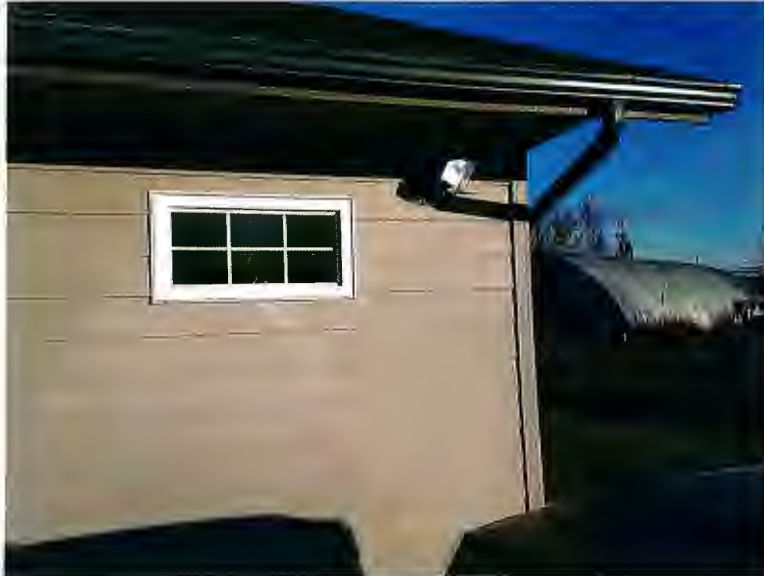
Photo 2: Light fixture needs second mounting screw.
