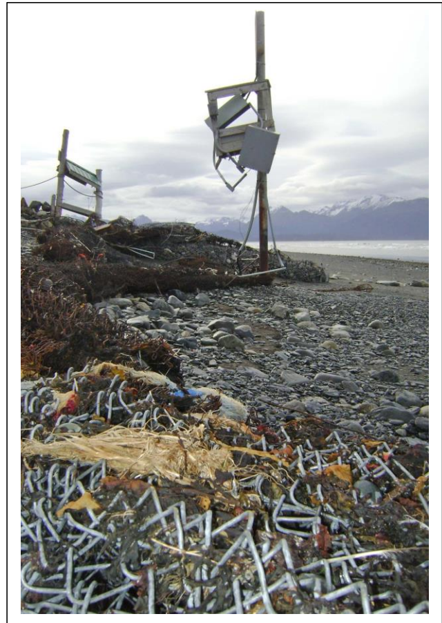
Thrashed gabions baskets and utilities are damaged by coastal storms.
