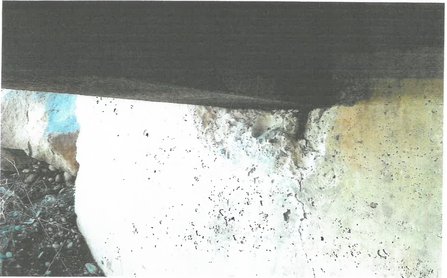
Garrison Ridge Road Bridge Concrete Scaling under SE end Beam # 2
