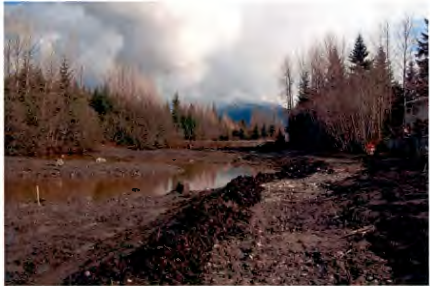
Glacier State shaped the rough trail bed and placed shot rock in May.
