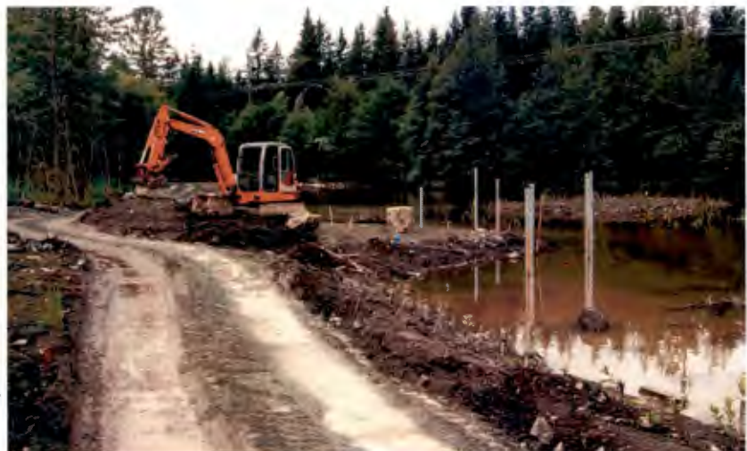
Trail Mix drives pilings for the observation deck and shapes the gathering area.
