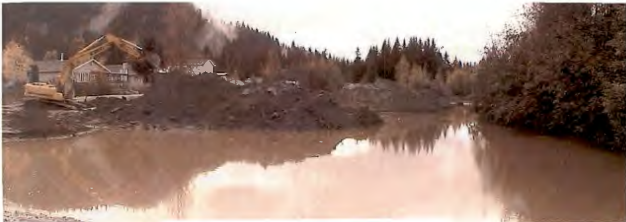
Early stages of filling in November, 2005. Photo looks south at the filling of the fingers. Photo taken by Alan Steffert.
