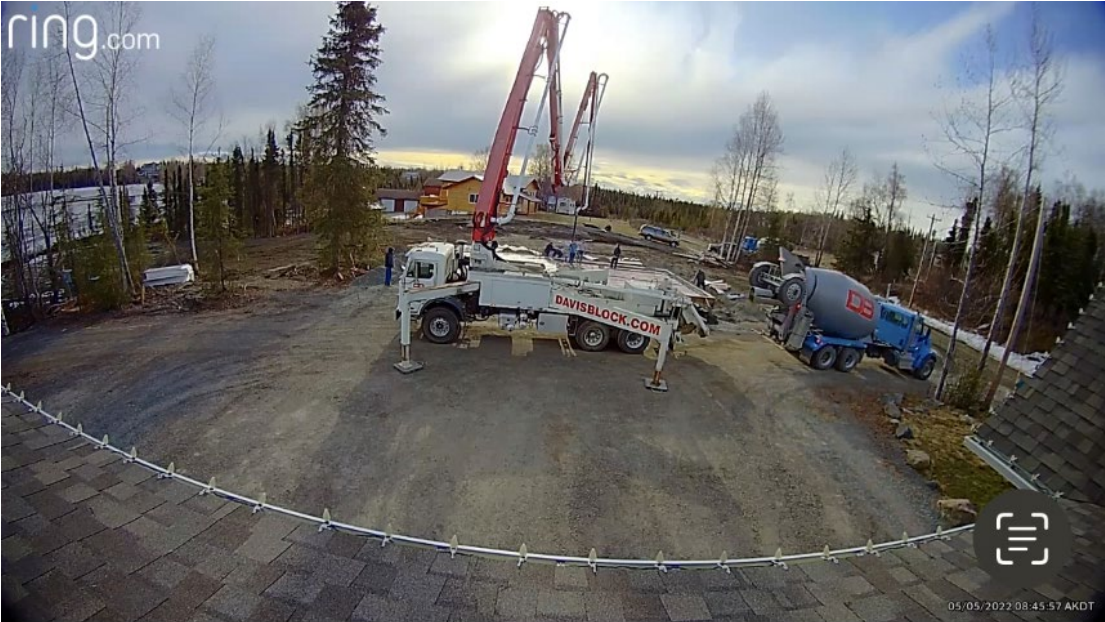
Attachment #1, Day one of pouring concrete for foundation, blocking access on GL Hollier.
