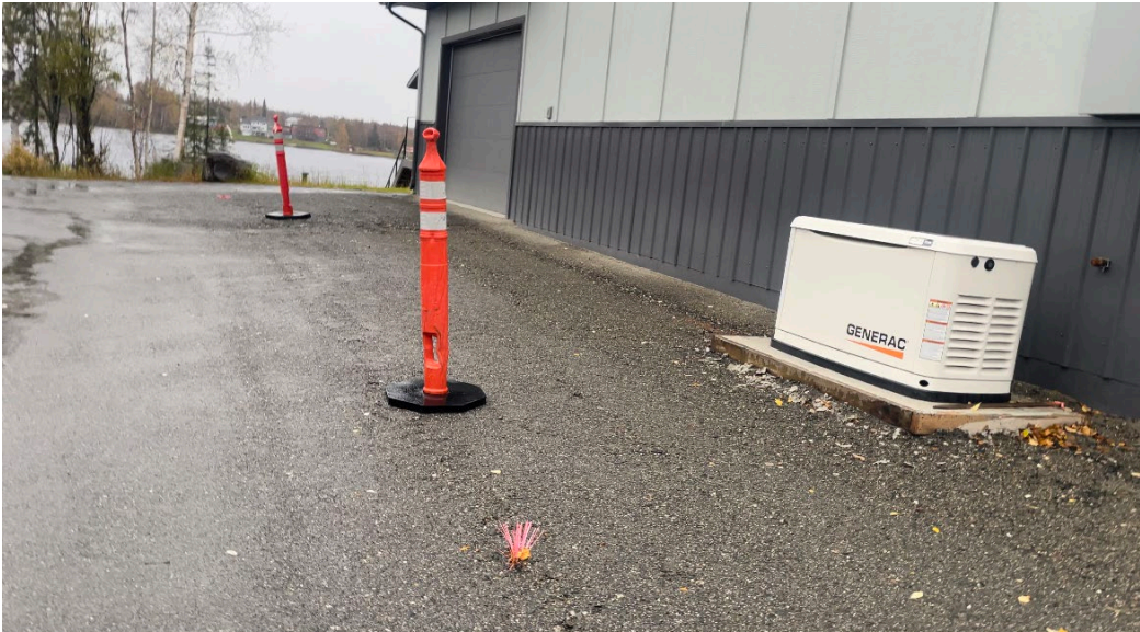
Attachment # 3, Generator beside shop in setback. The construction candle and whiskers depict the edge of the road.
