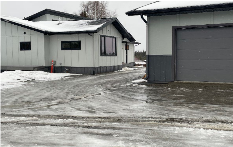
Attachment #11 Gutter draining into GL Hollier and creating gullies
