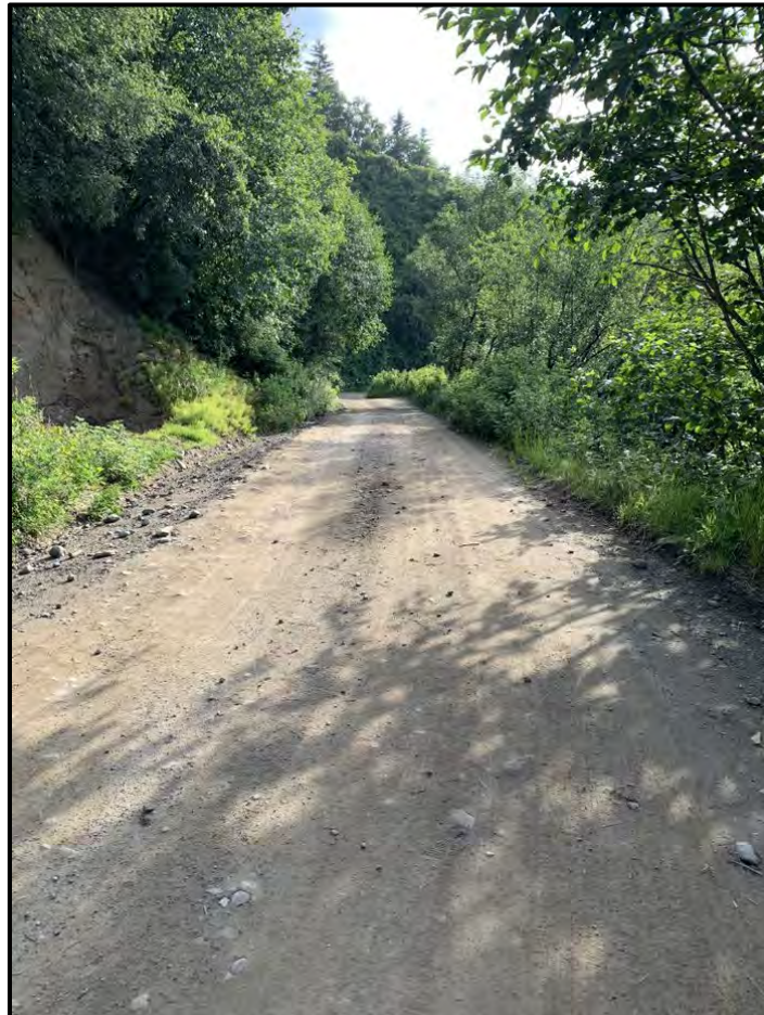
Figure 2.15. Narrow unpaved road that may make fire response difficult.
