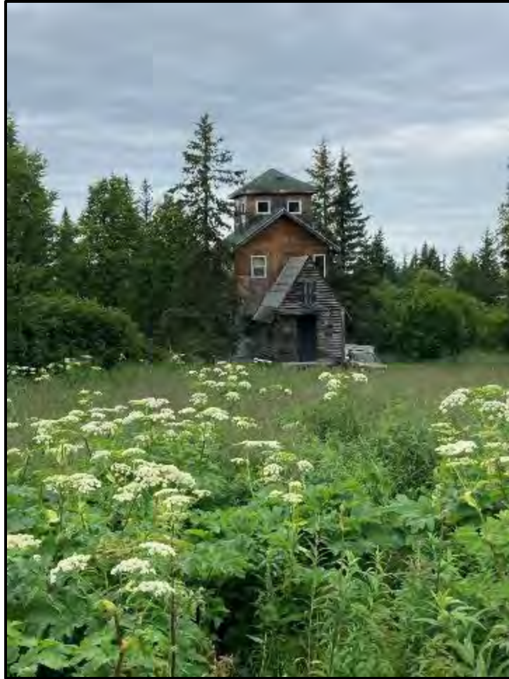
Figure D.26. Example of minimal yard maintenance contributing to hazardous fuels and poor defensible space.
